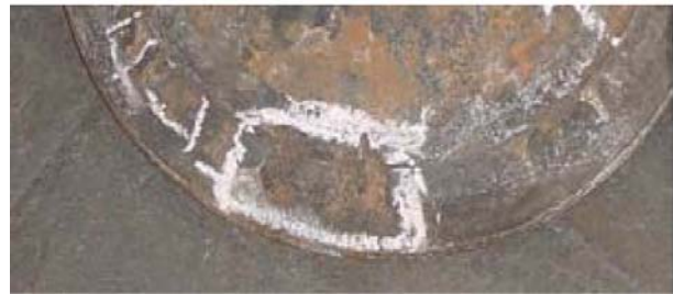
Figure 08: "Cobble stone corrosion" appearance of valve spindle failure through high-temperature corrosion (MC60 Standard-type)
